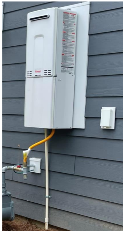
WATER HEATER Rianni Tankless Water Heater Exterior location temp control
